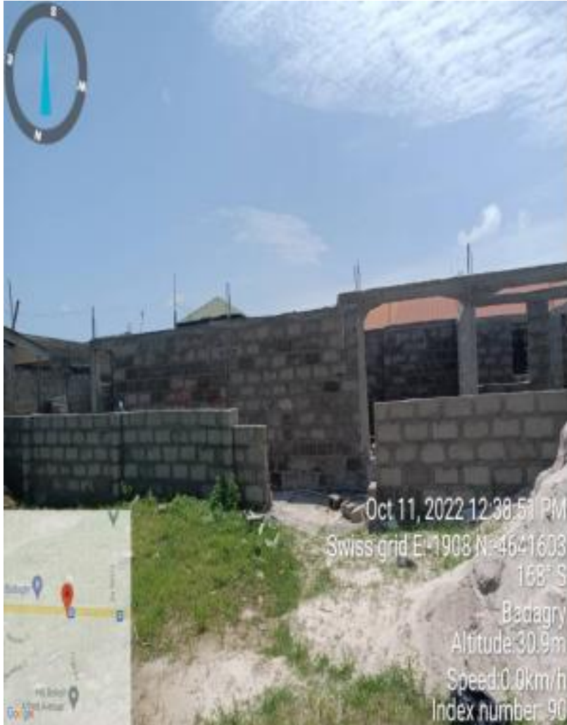
COMMERCIAL DEVELOPMENT AT LIMCA BUSTOP ALONG LAGOS BADAGRY EXPRESSWAY, OLORUNDA LCDA, BADAGRY
