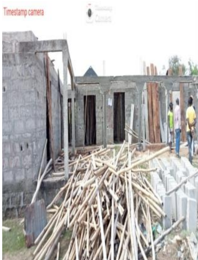
TWO FLOORS STRUCTURE UNDER CONSTRUCTION AT CHECKING POINT OPPOSITE TOLL PLAZA, ALONG LAGOS BADAGRY EXPRESSWAY OLORUNDA LCDA BADAGRY.
