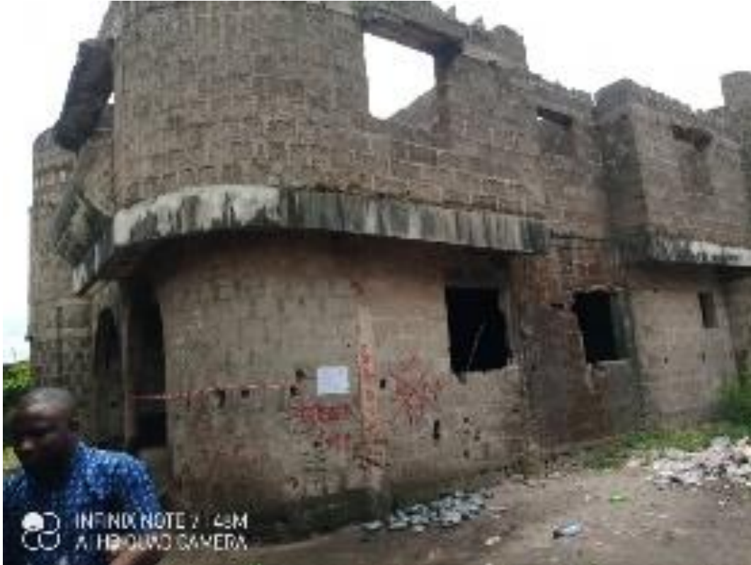
TWO FLOOR STRUCTURE ALONG CELE STRET, OFF LAGOS-BADAGRY EXPRESSWAY, MOROGBO OLORUNDA LCDA
