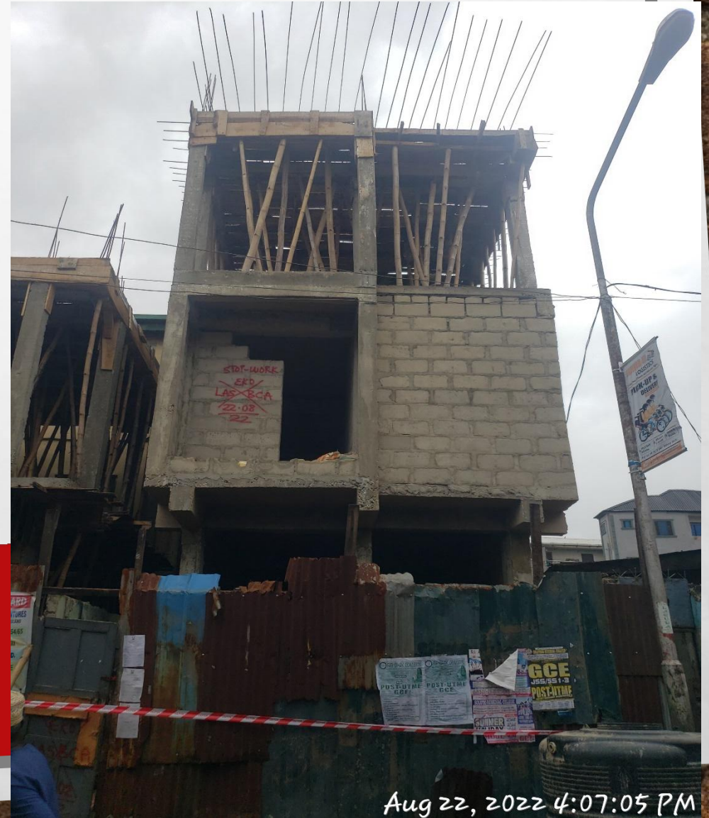
Location: 48, Glover Street, Lagos Island, Lagos. STAGE: THIRD SUSPENDED FLOOR SLAB REINFORCEMENT
