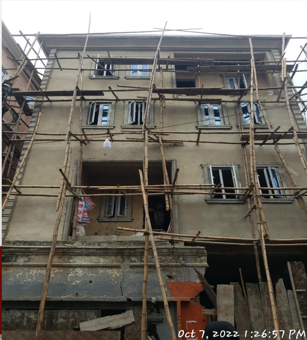
Location: 5, Inabere Street, Off Oshodi Street, Lagos Island, Lagos. STAGE: ROOFED AND PLASTERED
