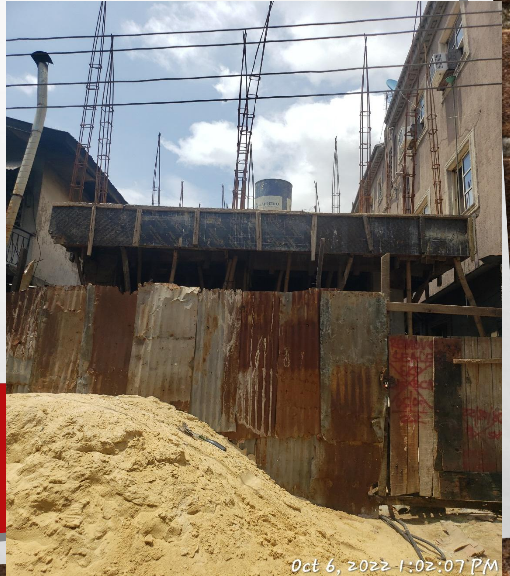
Location: 13, Osho Street, Lagos Island, Lagos. STAGE: FIRST SUSPENDED FLOOR COLUMN REINFORCEMENT
