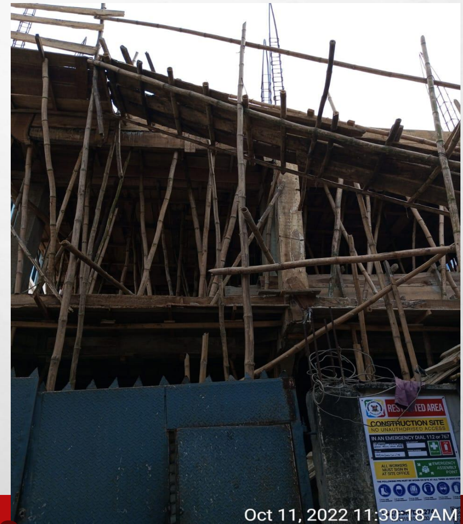
Location: 18 ABIBU OKI STREET OFF BROAD STREET , LAGOS ISLAND. Stage: THIRD FLOOR COLUMN
