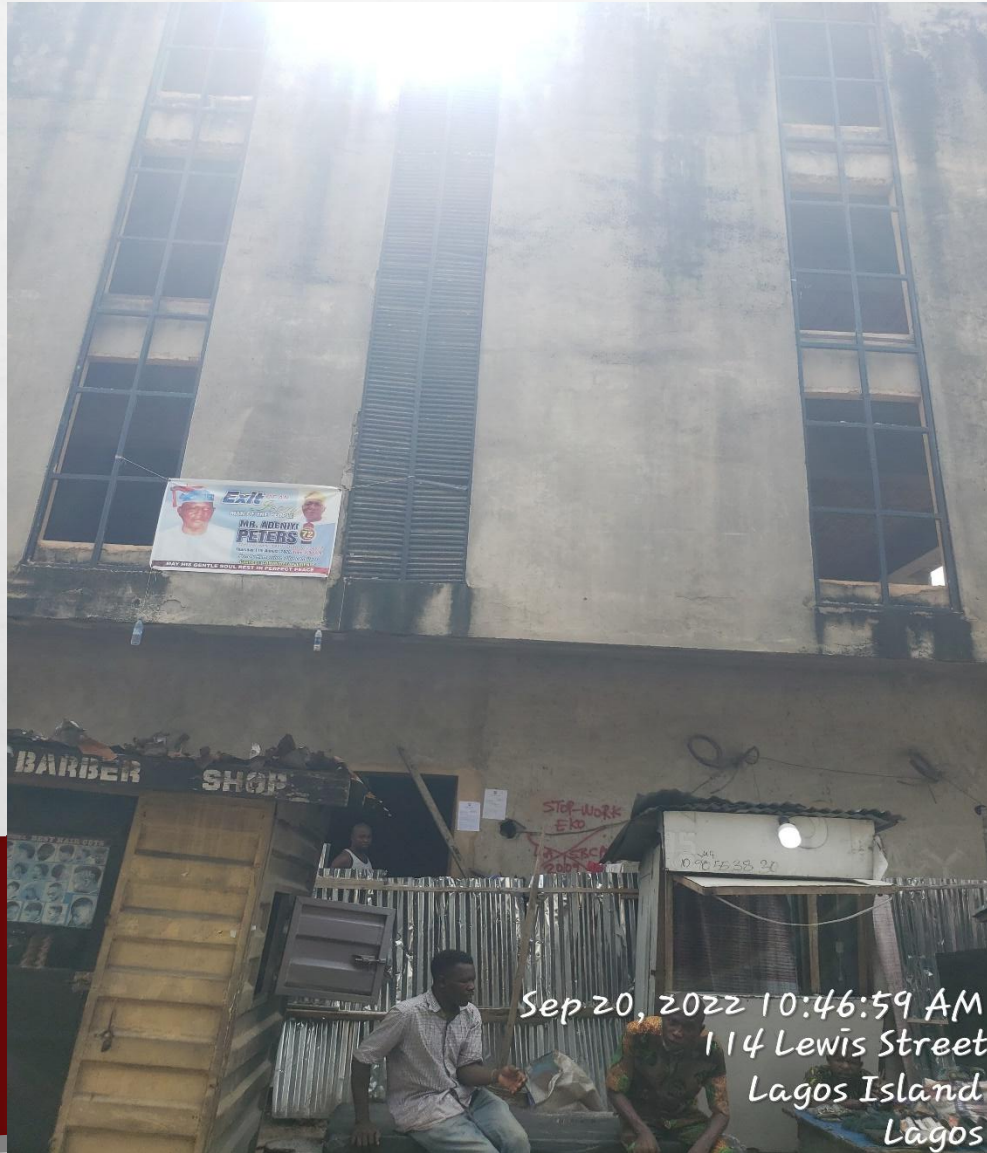
Location: Cornerpiece of Lewis Street by Hawley Street, Lagos. STAGE: FINISHES/BLOCK SETTING
