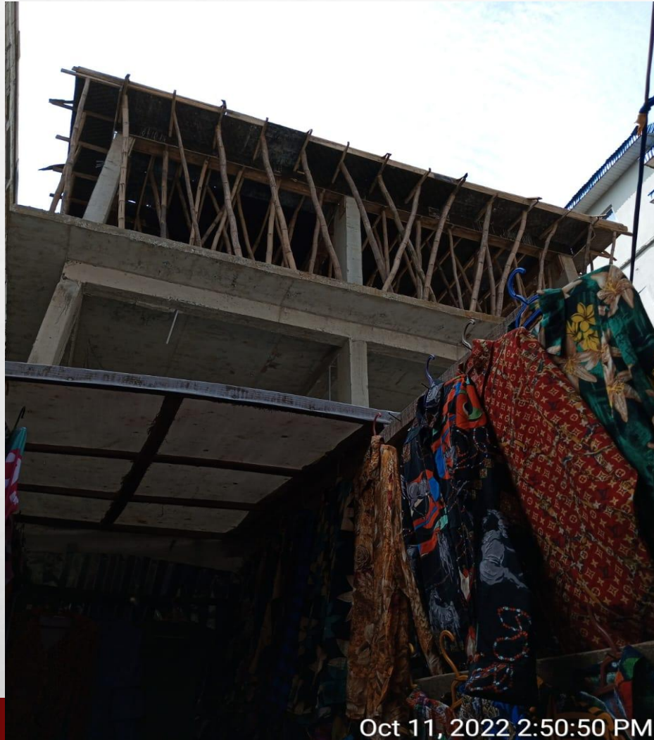
Location: 8 SANNI ADEWALE STREET , LAGOS ISLAND. Stage: THIRD SUSPENDED FLOOR SLAB FORMWORK
