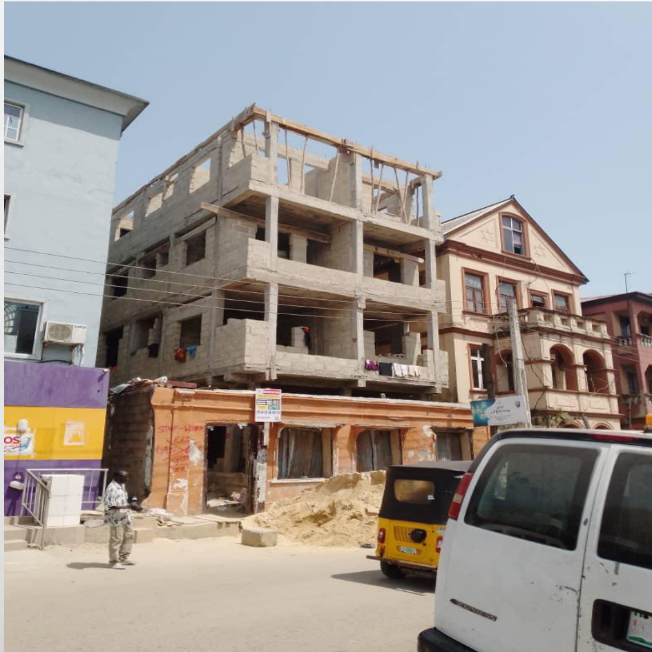
LOCATION: 19, IGBO SERE STREET, LAGOS ISLAND, LAGOS. STAGE: FOURTH FLOOR ROOF BEAM
