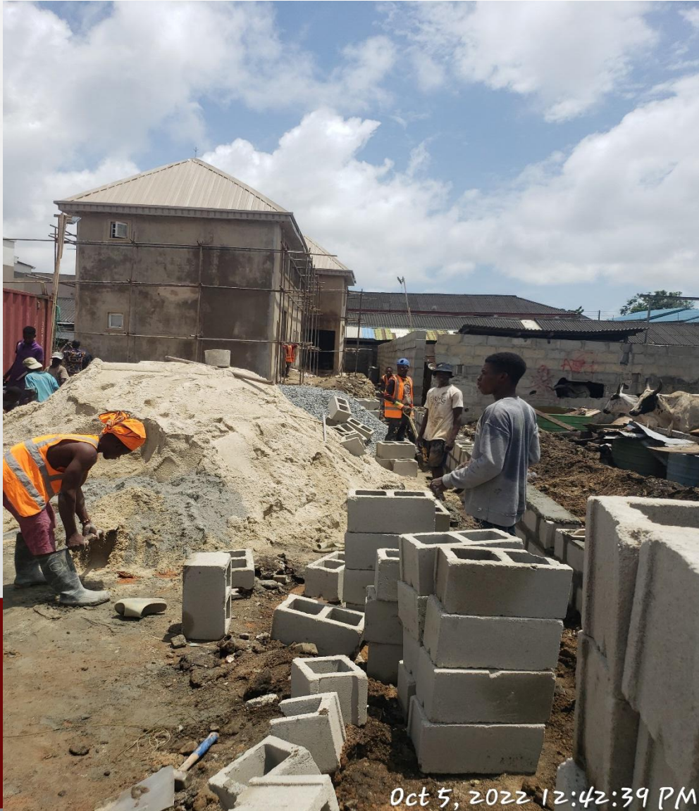
Location: Beside Total PFS, Along Simpson Street, Lagos Island, Lagos. STAGE: GROUND FLOOR (FOUNDATION)
