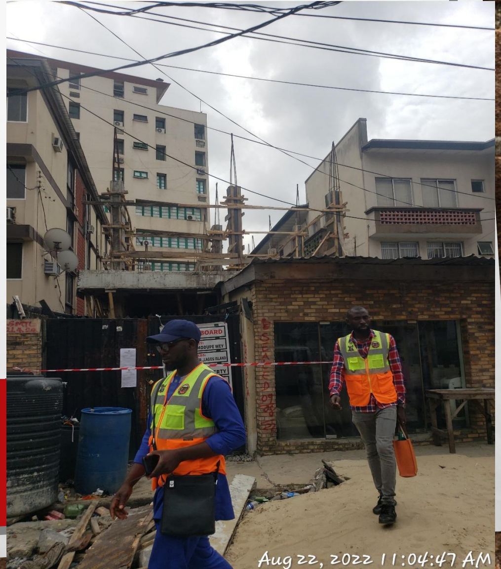
Location: 20, King George IV Street, Lagos Island, Lagos. STAGE: FIRST SUSPENDED FLOOR COLUMN
