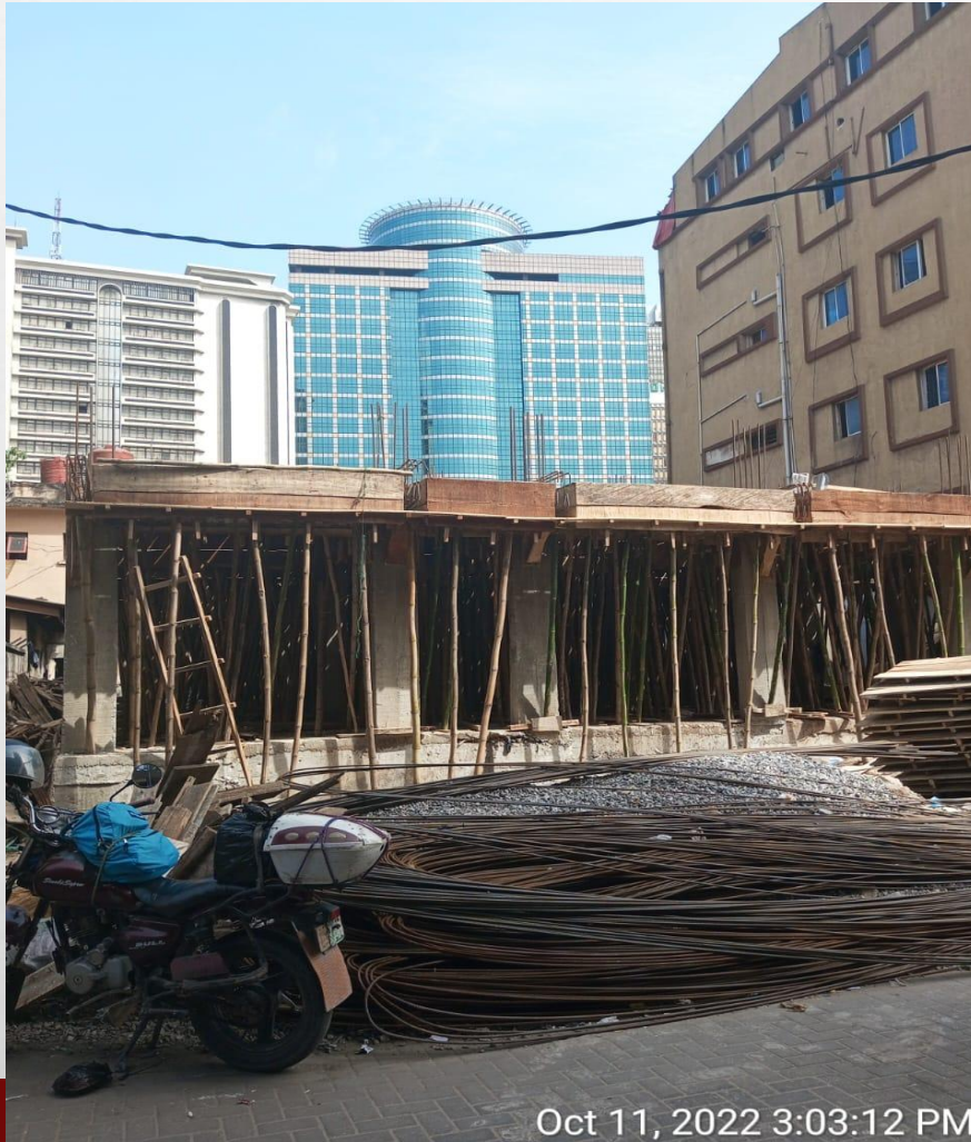
Location: 18 ABIBU OKI STREET OFF BROAD STREET , LAGOS ISLAND. Stage: FIRST FLOOR SLAB FORMWORK/REINFORCEMENT
