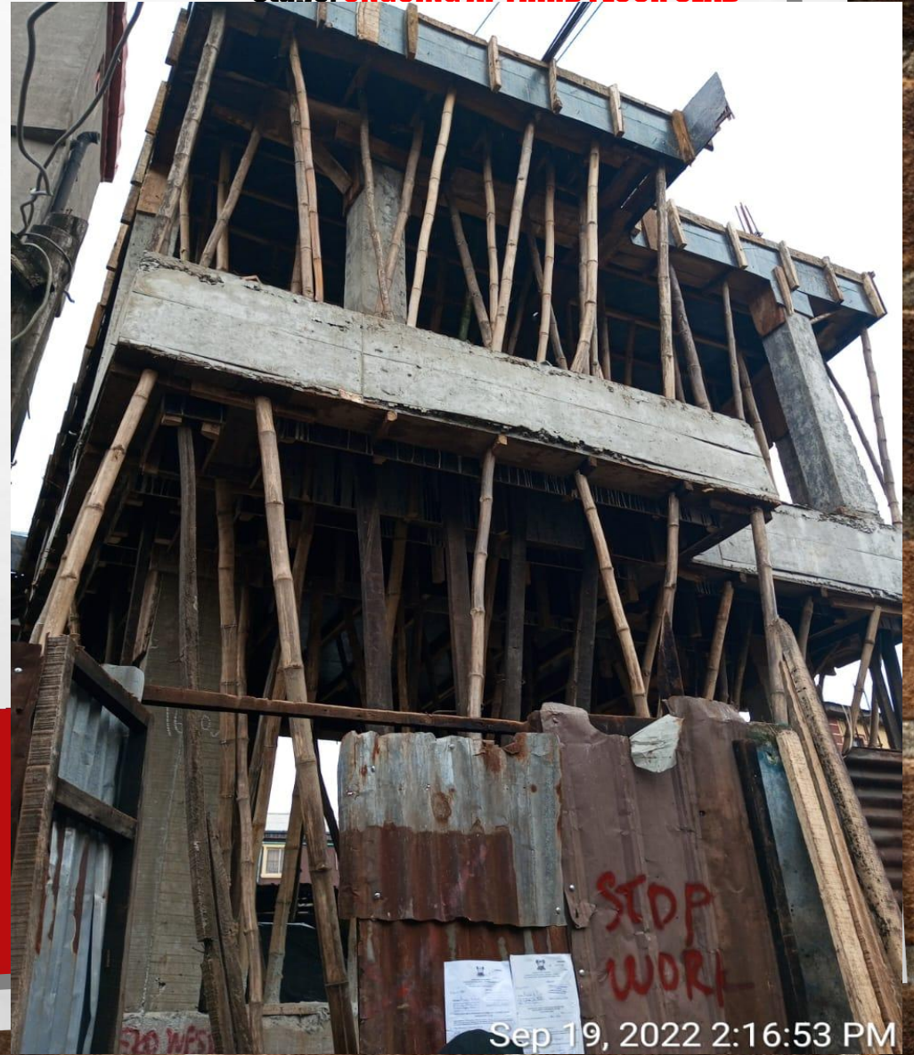
Location: 9, HASSAN LANE OFF AROLOYA STREET Stage: ONGOING AT THIRD FLOOR SLAB
