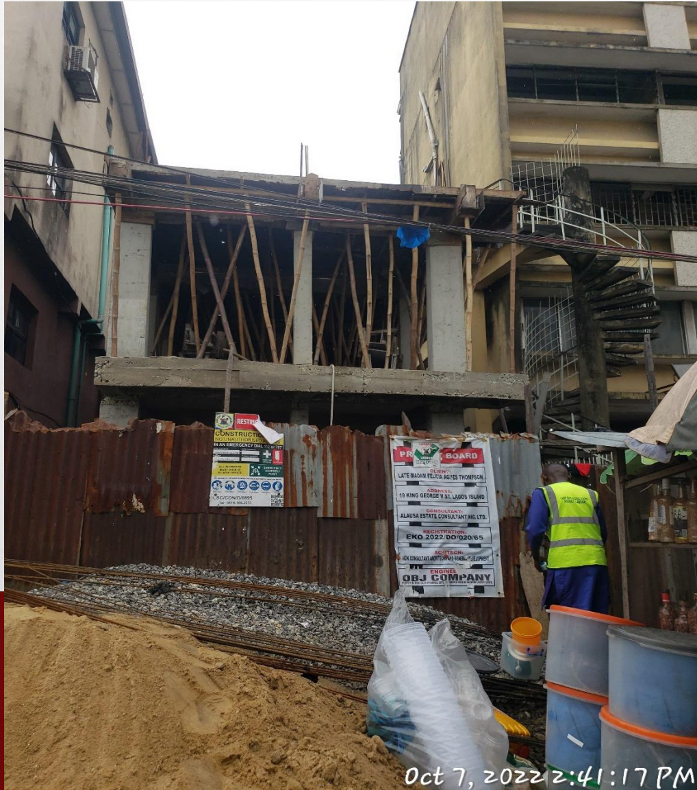
Location: 19, King George Street, Lagos Island, Lagos. STAGE: SECOND SUSPENDED FLOOR REINFORCEMENT
