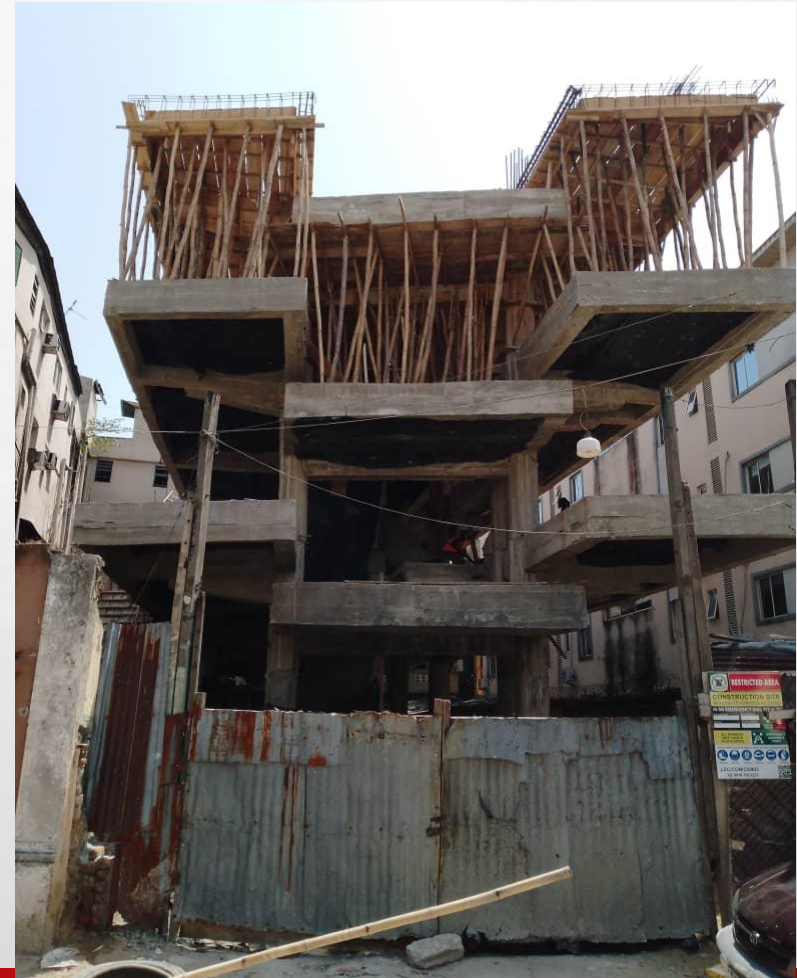
Location: UPPER CAMPUS, ALONG AJELE Street, Lagos Island, Lagos. STAGE: Third suspended floor formwork
