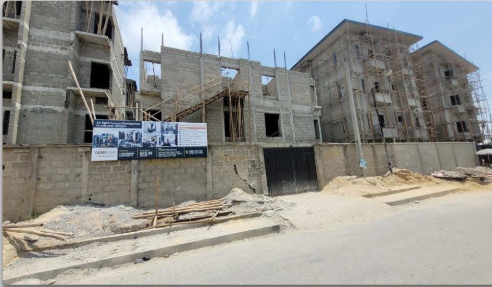
CONSTRUCTION OPPOSITE THE ADDRESS HOMES, ILASAN NEW ROAD, LEKKI APPROVAL STATUS- NOT ASCERTAINED NO OF FLOORS- 3 FLOORS
