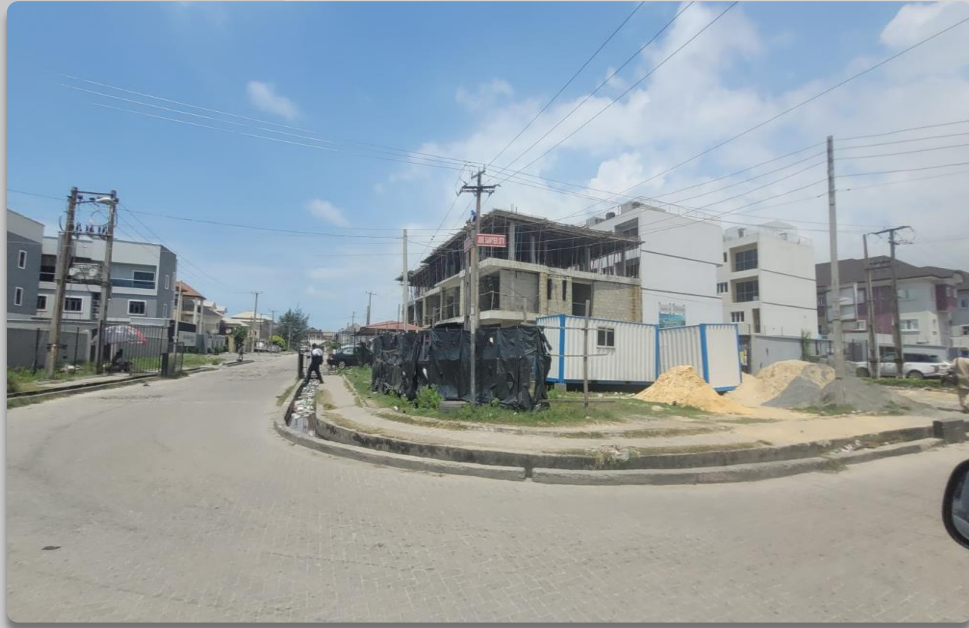
4 FLOOR STRUCTURE ALONG JIDE SAWYER BY ADEKOLA BALOGUN STREET, LEKKI 1 APPROVAL STATUS- APPROVED NO OF FLOORS- 4 FLOORS
