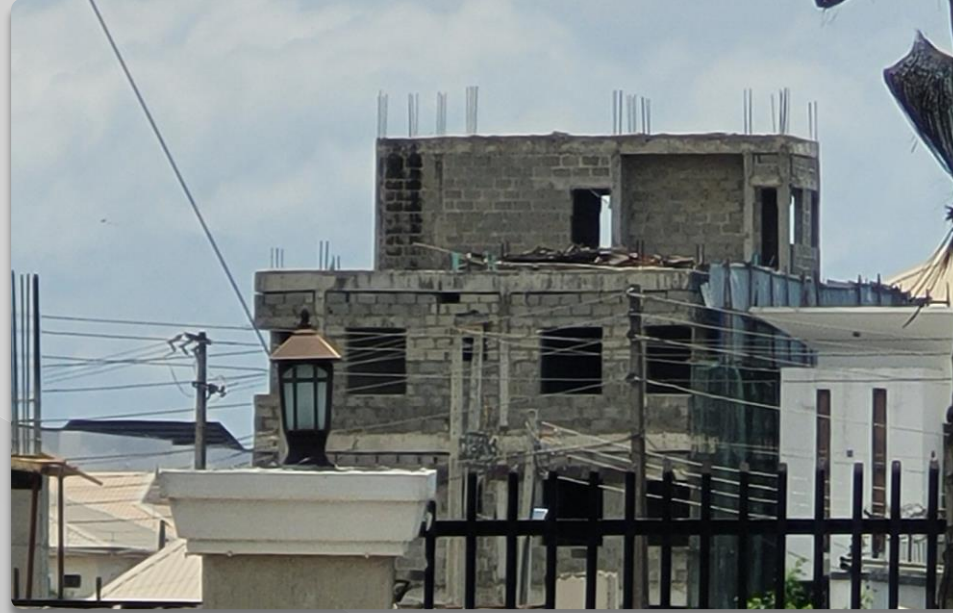
PROPERTY ALONG TOBI LAWAL STREET OLOGOLO APPROVAL STATUS- NOT ASCERTAINED NO OF FLOORS- 4 FLOORS
