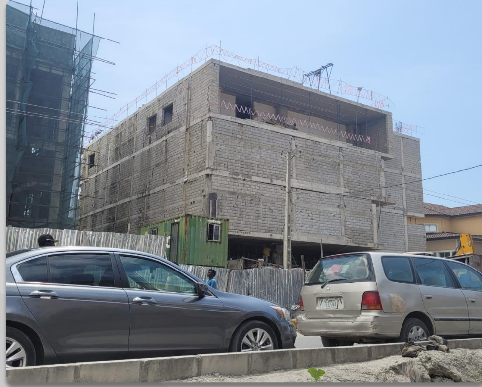
4 FLOOR STRUCTURE OPPOSITE ONIRU ESTATE ALONG AKIOGUN ROAD, LEKKI APPROVAL STATUS- APPROVED STAGE CERTIFICATION - ONGOING NO OF FLOORS- 4 FLOORS
