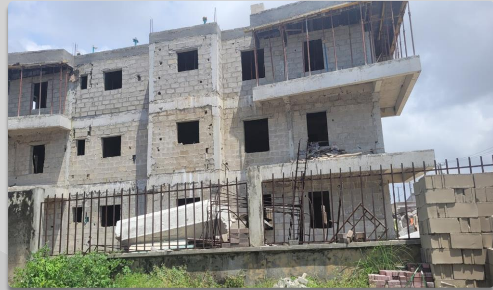
4 FLOOR STRUCTURE ALONG HAKEEM DICKSON STREET BY BOSUN ADEKOYA STREET. APPROVAL STATUS- NOT ASCERTAINED NO OF FLOORS- 4 FLOORS
