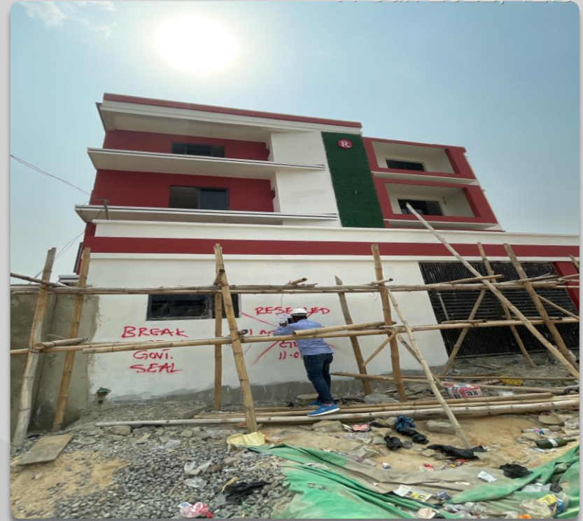
PROPERTY ALONG OLOGOLO STREET OFF ALHAJI TOLANI STREET, OLOGOLO APPROVAL STATUS- UNKNOWN. NO OF FLOORS- 3 FLOORS
