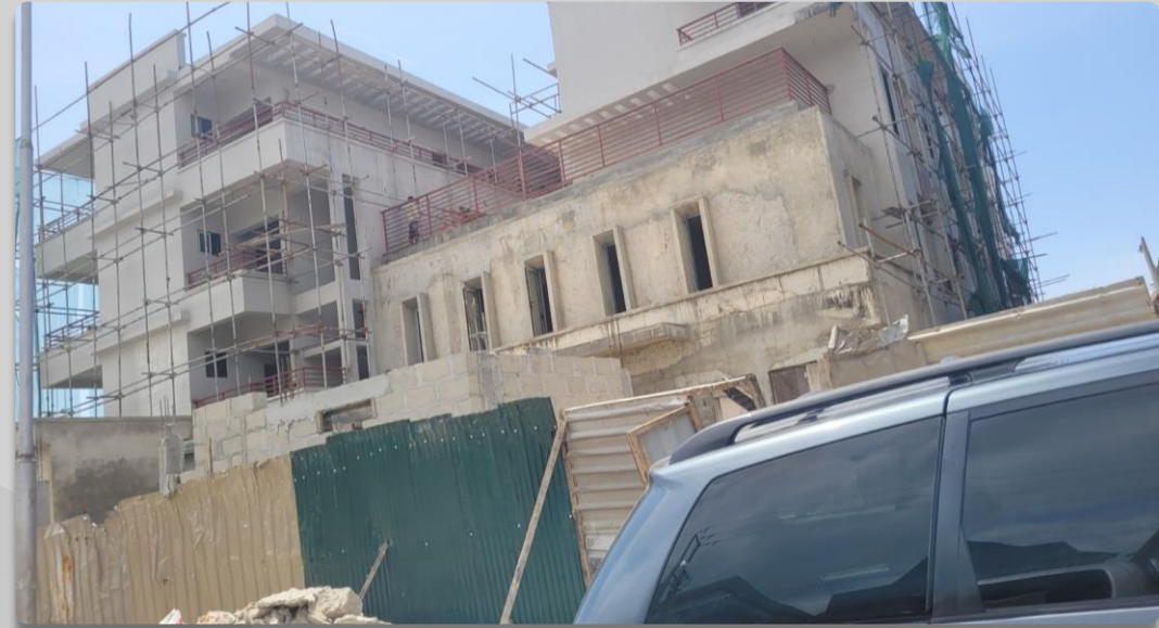
4 FLOOR STRUCTURE ALONG BOSUN ADEKOYA, LEKKI 1. APPROVAL STATUS- NOT ASCERTAINED NO OF FLOORS- 4 FLOORS
