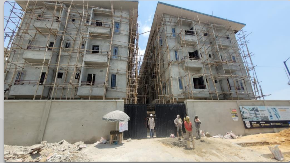
4 FLOOR CONSTRUCTION ALONG ILASAN NEW ROAD. APPROVAL STATUS- APPROVED NO OF FLOORS- 4 FLOORS
