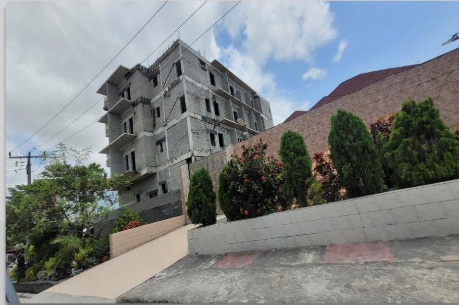
JOSE MARIA 5 FLOORS, BESIDE NIKE ART GALLERY APPROVAL STATUS- NOT ASCERTAINED NO OF FLOORS- 5 FLOORS
