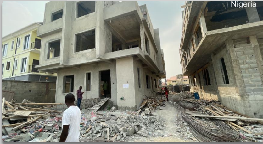
PROPERTY ALONG EDWARD HOTONU STREET BEHIND UPDC ESTATE LEKKI PHASE 1 APPROVAL STATUS- UNKNOWN. NO OF FLOORS- 3 FLOORS
