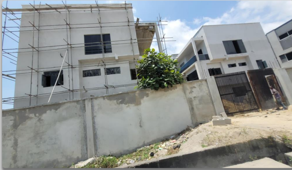
CONSTRUCTION BESIDE THE ADDRESS HOMES, ILASAN NEW ROAD, LEKKI APPROVAL STATUS- NOT ASCERTAINED NO OF FLOORS- 3 FLOORS
