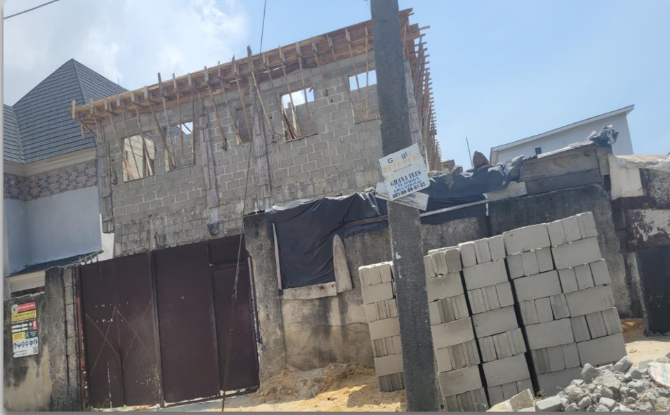
2 FLOOR STRUCTURE ALONG HAKEEM DICKSON OPPOSITE WALTON PARK RESIDENCE APPROVAL STATUS- NOT ASCERTAINED NO OF FLOORS- 2 FLOORS
