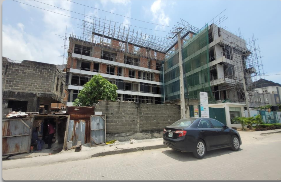
DELE OGUNBOWALE CRESCENT APPROVAL STATUS- EPN 2021/ ETO/311W STAGE CERTIFICATION – ONGOING NO OF FLOORS- 6 FLOORS
