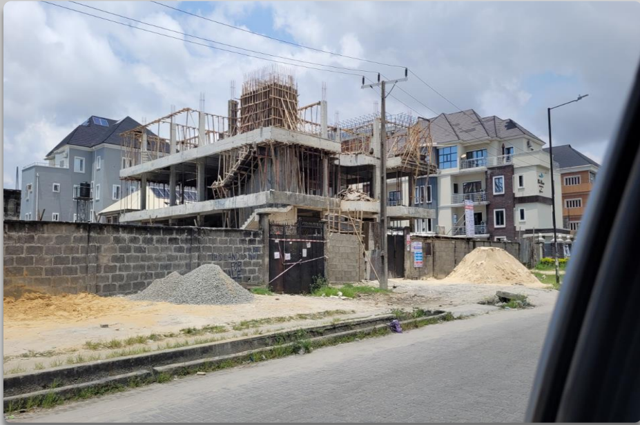
PROPERTY ALONG JOSE MARIA AKINYEMI AVENUE APPROVAL STATUS- REG NO EPN/2020/ETO/0279 NO OF FLOORS- 3 FLOORS
