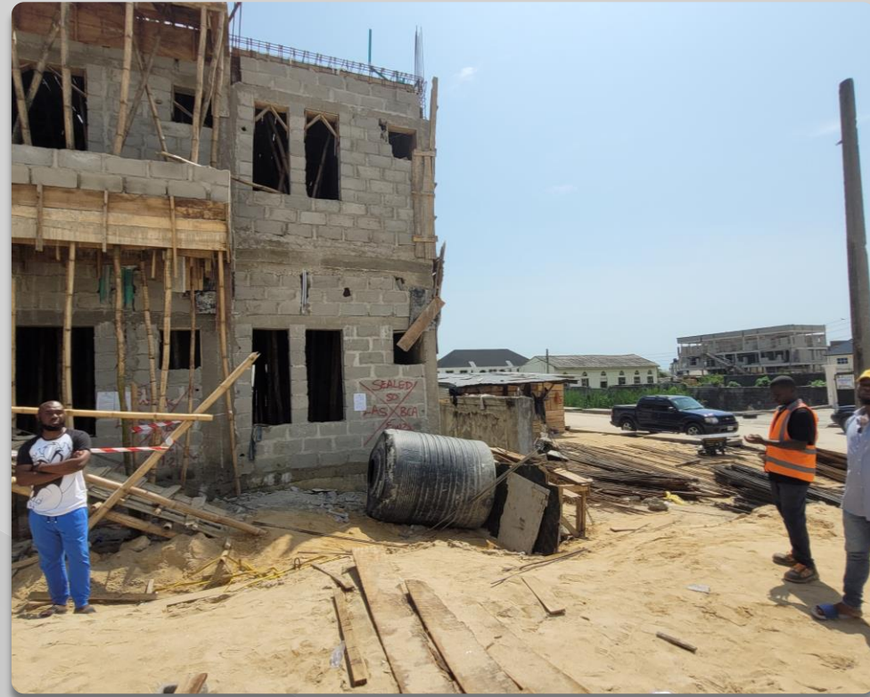
PROPERTY AT THE CORNERPIECE OF OLOGOLO ROAD AND CHIEF KOLA OLOGOLO STREET, OLOGOLO. APPROVAL STATUS- IN PROGRESS. NO OF FLOORS- 2 FLOORS
