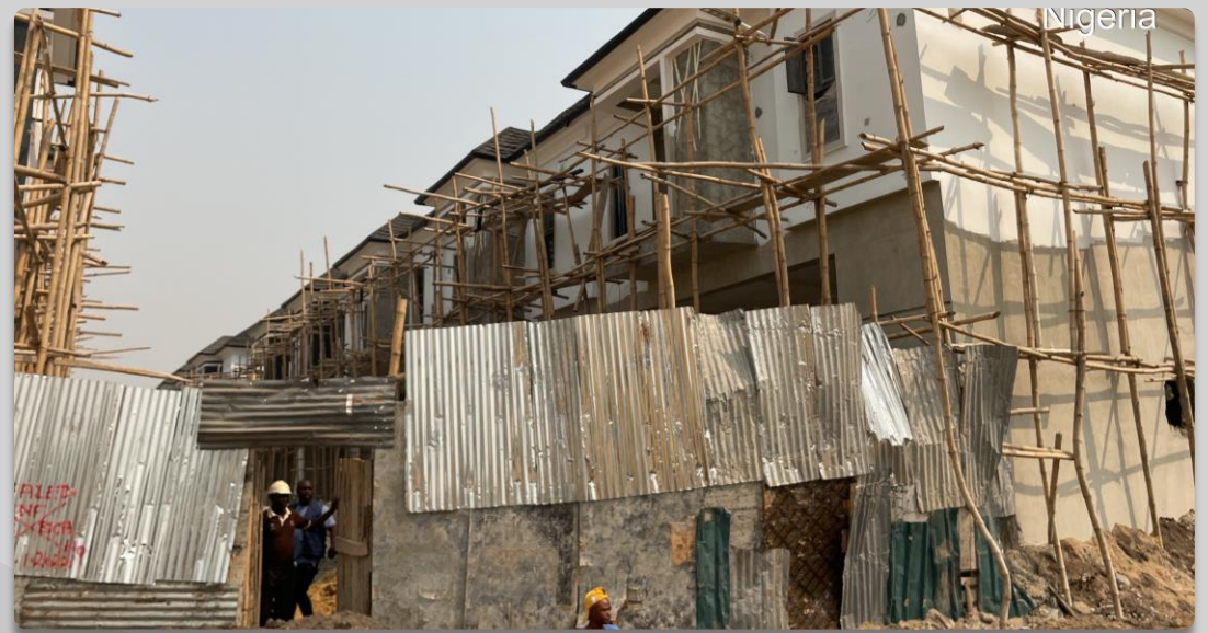
PROPERTY ALONG AN EXISTING ROAD OFF OGA NDI OGA STREET OFF ORCHID ROAD APPROVAL STATUS- UNKNOWN. NO OF FLOORS- 2 FLOORS
