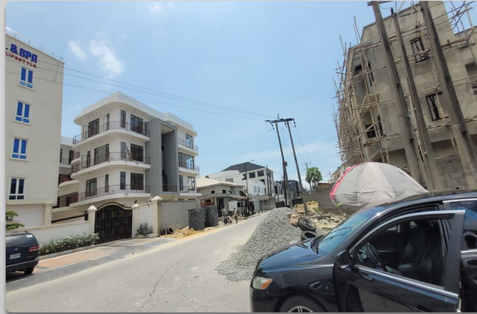
JOSE MARIA BY WHITE SANDS, 4 FLOORS APPROVAL STATUS- NOT ASCERTAINED NO OF FLOORS- 4 FLOORS
