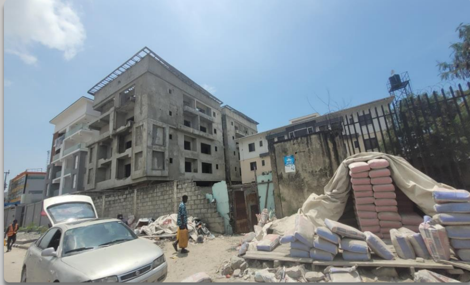
CONSTRUCTION OF 4 FLOORS BESIDE QMB BUILDERS MART ALONG QMB ROAD. APPROVAL STATUS- NOT ASCERTAINED NO OF FLOORS- 4 FLOORS
