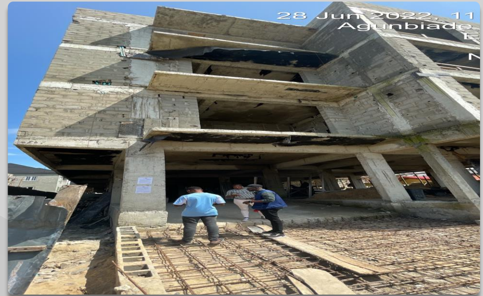
PROPERTY ALONG AGUNBIADE STREET OLOGOLO APPROVAL STATUS- UNKNOWN. NO OF FLOORS- 4 FLOORS
