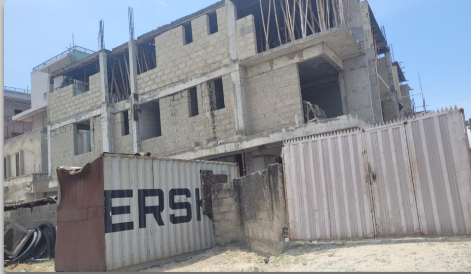
3 FLOOR STRUCTURE ALONG BOSUN ADEKOYA, LEKKI 1 APPROVAL STATUS- NOT ASCERTAINED NO OF FLOORS- 3 FLOORS
