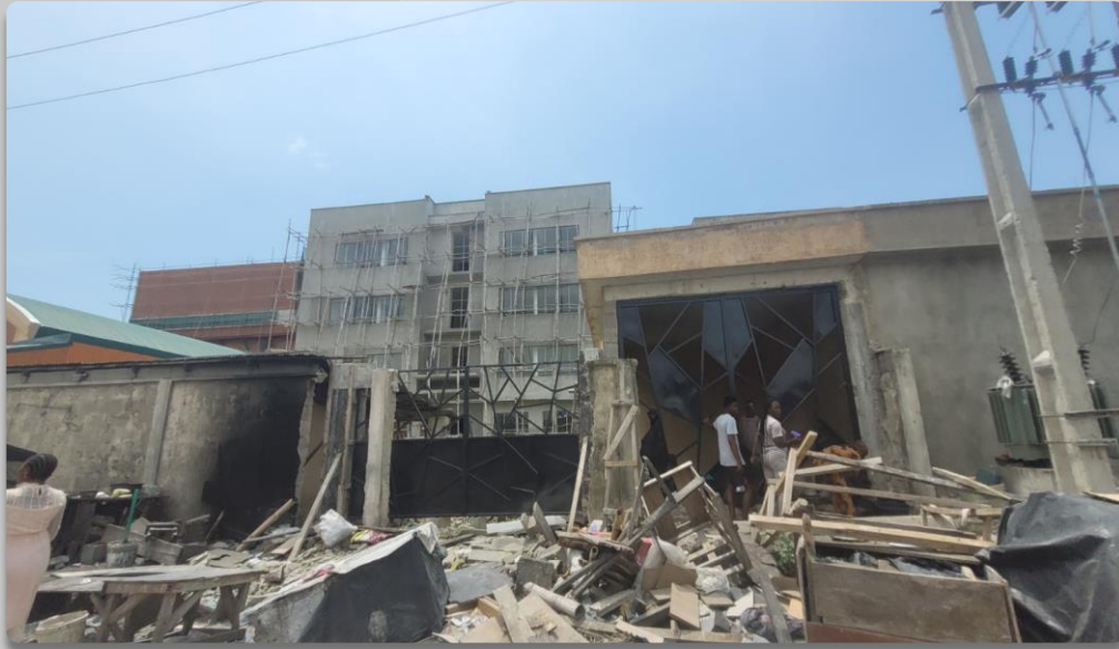
4 FLOOR CONSTRUCTION BY QMB MART APPROVAL STATUS- NOT ASCERTAINED NO OF FLOORS- 4 FLOORS
