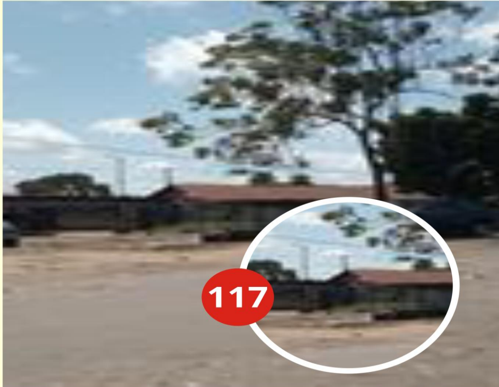
ADDRESS OF PROPERTY: OLD LAGOS ROAD, AFOYONDE, TORIKOH, AJARA, BADAGRY DESCRIPTION OF PROPERTY: BUNGALOW STAGE OF WORK: ROOFED DATE CAPTURED: 6TH OCTOBER 2022
