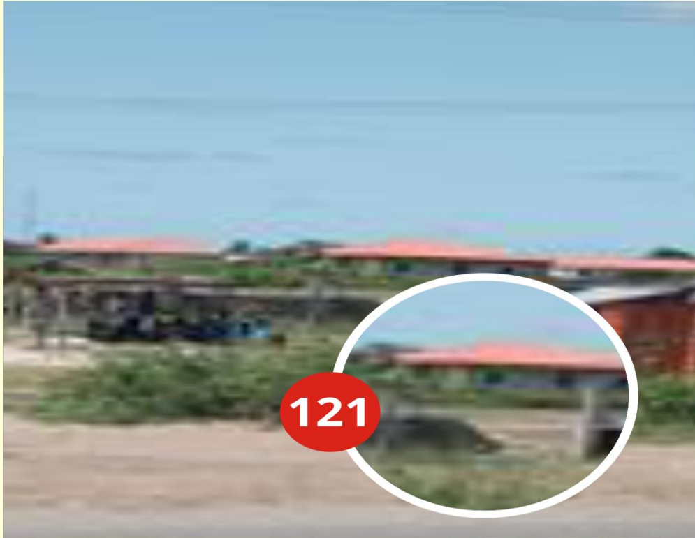
ADDRESS OF PROPERTY: FEDERAL YOUTH CENTER ALONG LAGOS-BADAGRY EXPRESSWAY BADAGRY DESCRIPTION OF PROPERTY: MULTIPLE BUNGALOWS STAGE OF WORK: ROOFED DATE CAPTURED: 6 TH OCTOBER 2022
