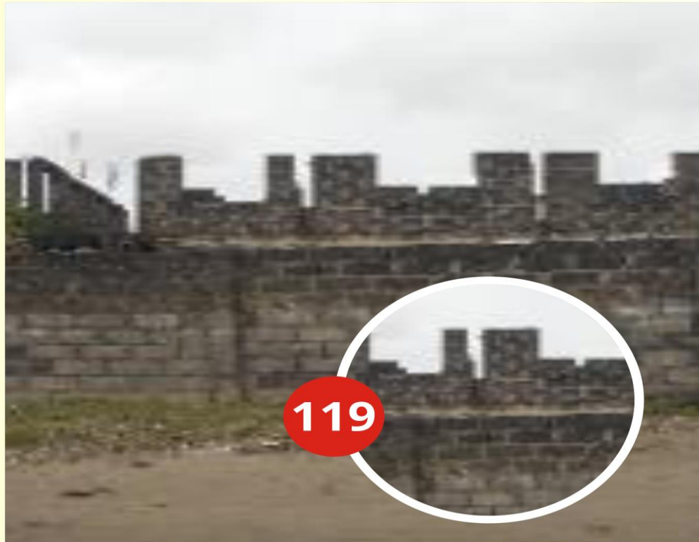
ADDRESS OF PROPERTY: ALONG SEJE ROAD, BEHIND SYCOMORE HOTEL, AJARA TOPA, BADAGRY DESCRIPTION OF PROPERTY: 2 FLOORS STAGE OF WORK: WINDOW LEVEL DATE CAPTURED: 6 TH OCTOBER 2022
