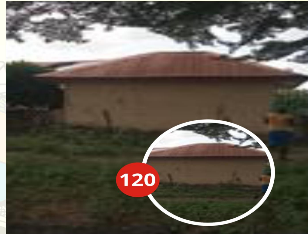
ADDRESS OF PROPERTY: ALONG DOKOH ROAD, AJARA, BADAGRY DESCRIPTION OF PROPERTY: BUNGALOW STAGE OF WORK: ROOFED DATE CAPTURED: 6 TH OCTOBER 2022
