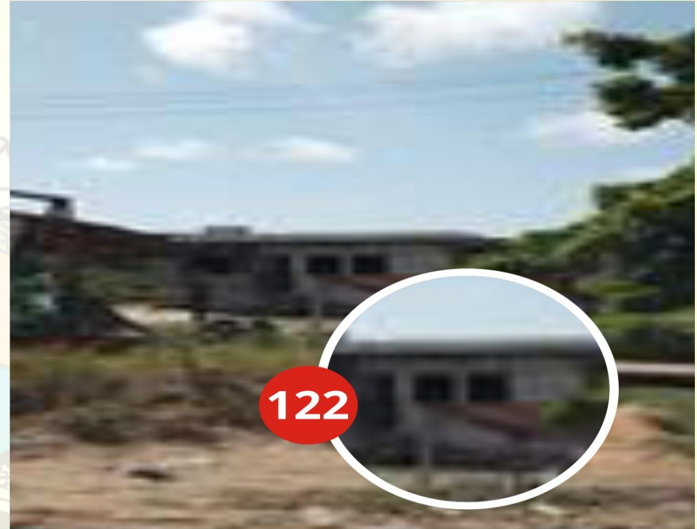
ADDRESS OF PROPERTY: ALONG LAGOS BADAGRY EXPRESSWAY BADAGRY DESCRIPTION OF PROPERTY: BUNGALOW STAGE OF WORK: ROOFED DATE CAPTURED: 6 TH OCTOBER 2022
