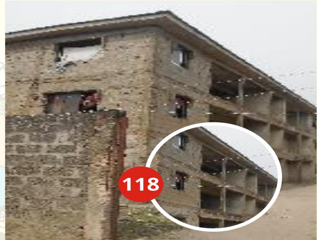
ADDRESS OF PROPERTY: HARMONY SANCTUARY BEHIND GALERIA PLAZA OFF SEME ROAD, BADAGRY DESCRIPTION OF PROPERTY: 3 FLOORS STAGE OF WORK: ROOFED DATE CAPTURED: 6TH OCTOBER 2022
