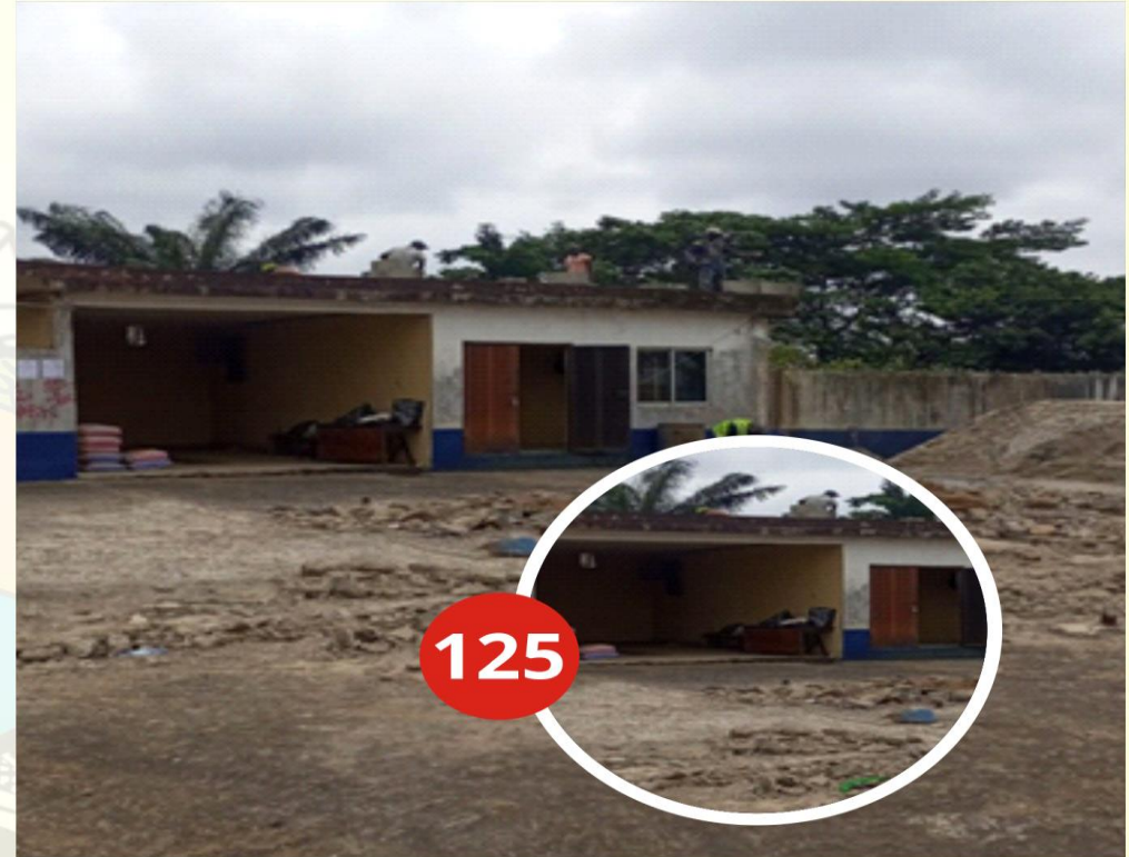
ADDRESS OF STRUCTURE: PFS UNDER RENOVATION ALONG AVIA ROAD, BADAGRY DATE CAPTURED:22/08/2022
