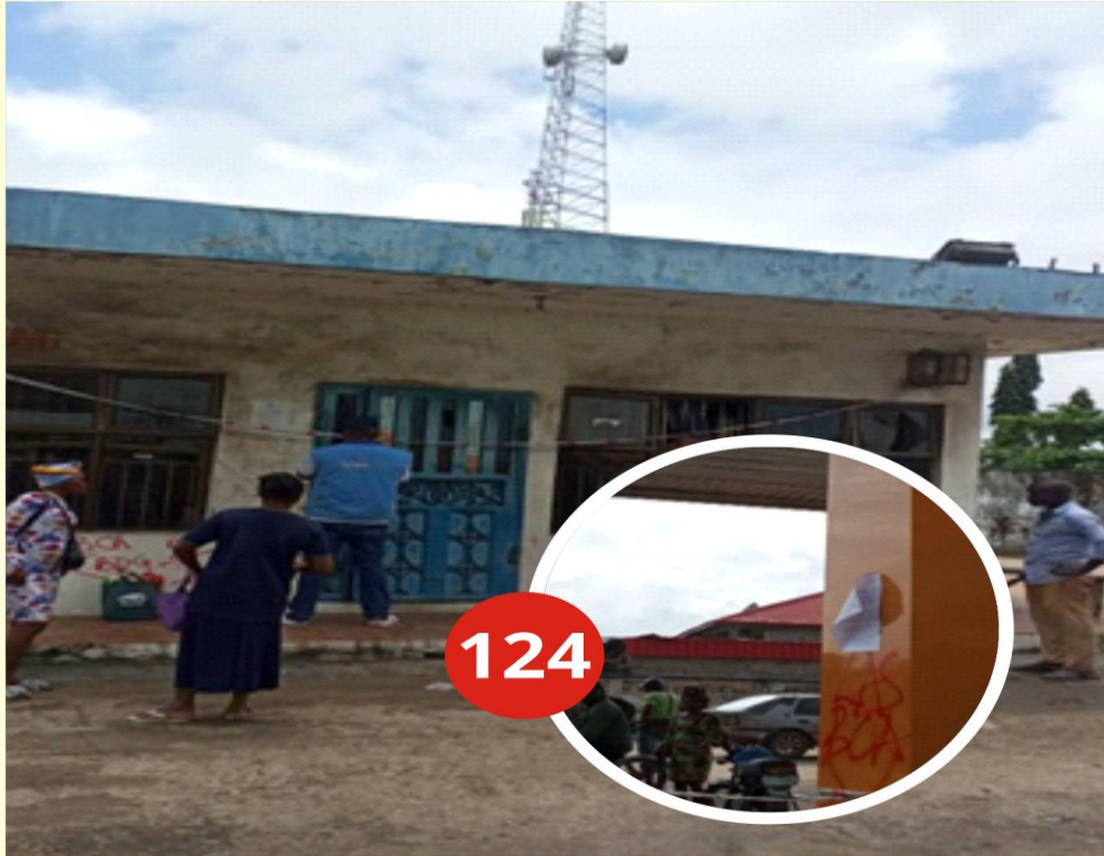
ADDRESS OF STRUCTURE: ASCON OIL UNDER RENOVATION ALONG LAGOS-BADAGRY EXPRESSWAY, ROUNDAABOUT, BADAGRY DATE CAPTURED:07/10/2022
