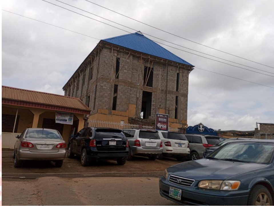
48. THE REDEEMED CHRISTIAN CHURCH OF GOD BESIDE FORTE OIL GATE BUS STOP ALONG 21 ROAD
