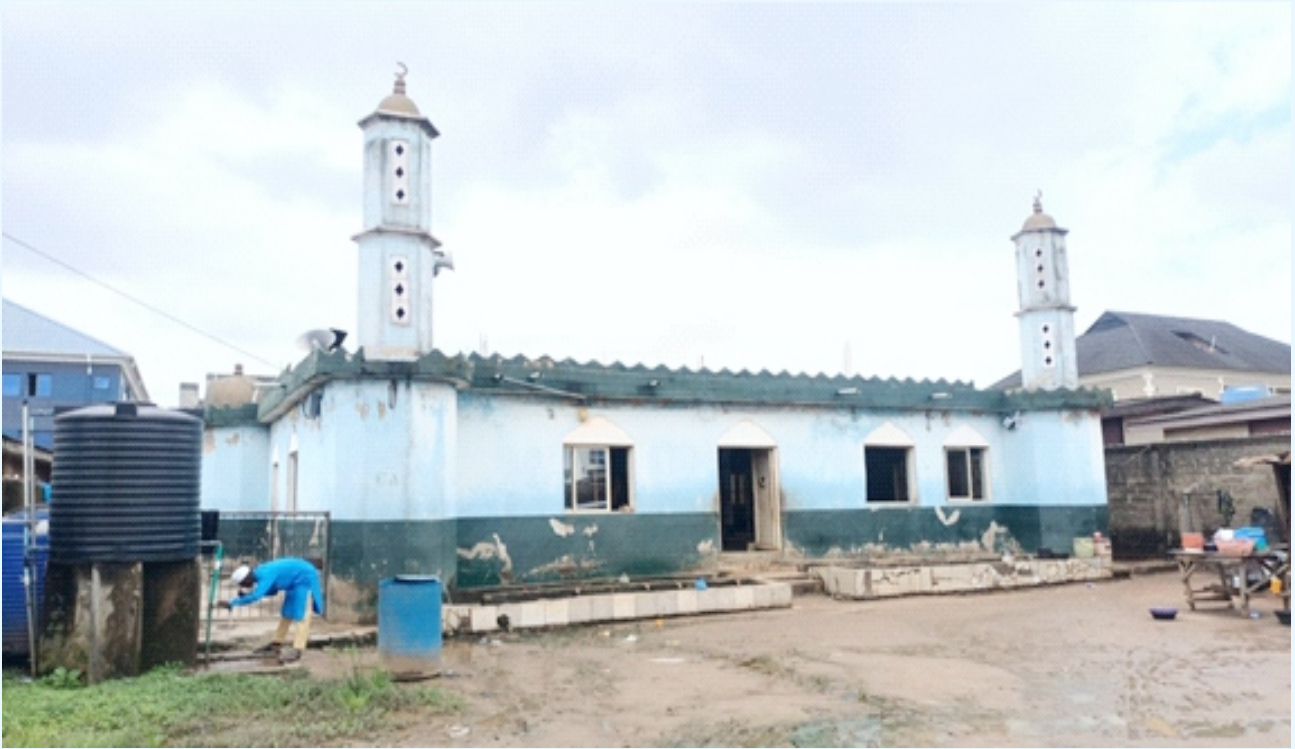
BAHSOA MOSQUE ALONG ASHIPA ROAD 6, BAHRU ULOOMY CLOSE, ASHIPA ROAD, AMULE BUS-STOP, MEGIDA AYOBO. BUNGALOW WITH VISIBLE SIGNS OF DAMPNES.
