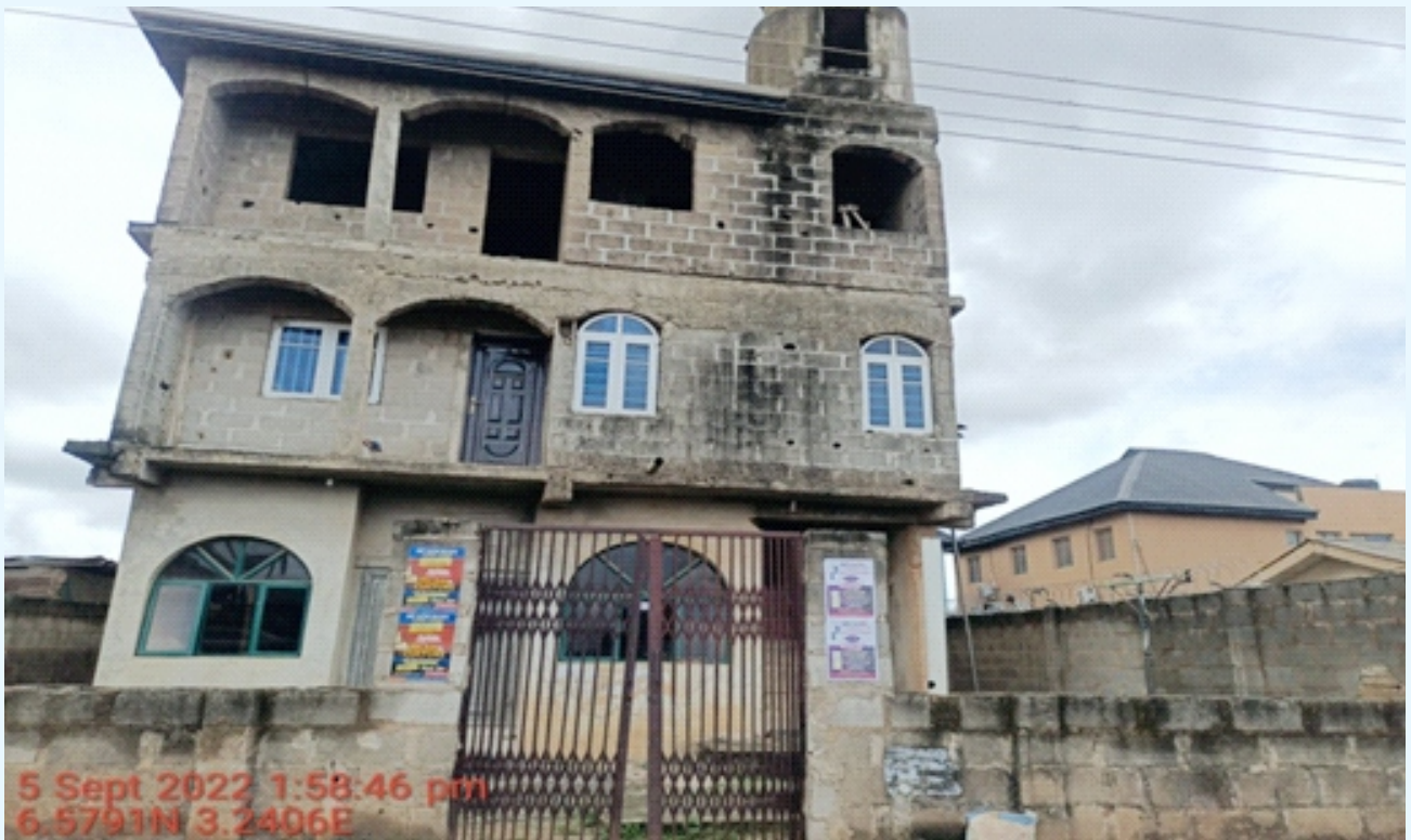
QMP RATIBI MOSQUE 3-FLOORS, 2 ALABI ASHIPA ROAD, OLAYEMI, AYOBO. ROOFED AND UNPLASTERED
